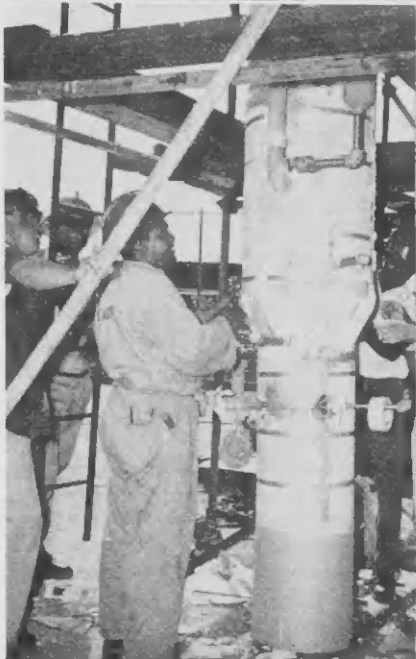
FEW MINUTES after pouring, cardboard is removed and foam is allowed to harden. Foam area is covered, completing the insulation. POCO MINUUT despues di basha, e carton ta ser kitá y e scuma ta worde permiti pa bira duro. E scuma seco luego ta worde tapá tur rond, completando e insulacion.
